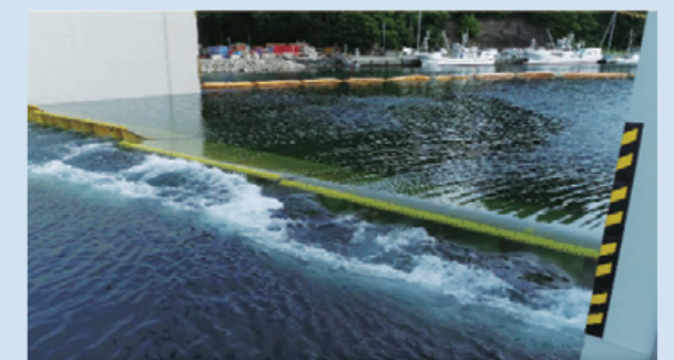
Seabed-mounted flap-gate type seawall for Iwate Prefecture (gate floating: from outside the harbor)
