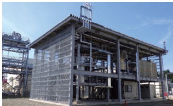
Methanation test facility
