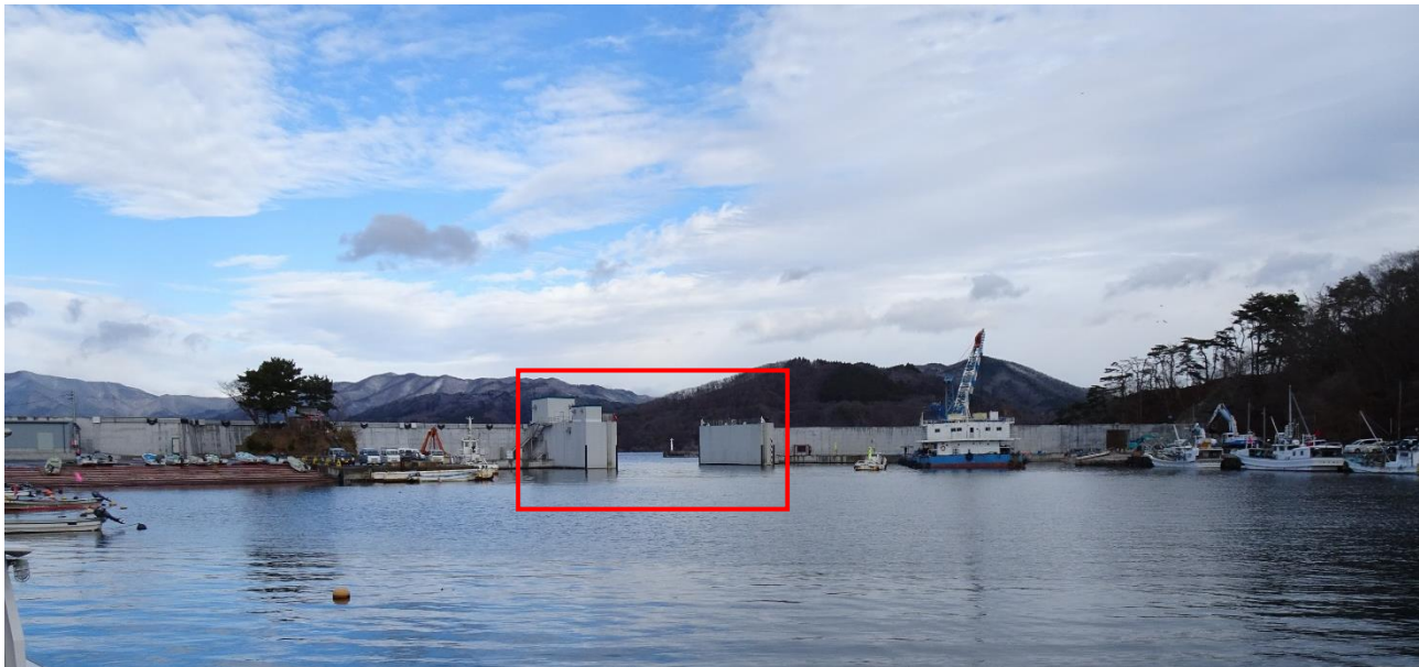
Implementation case at the Hosoura area of Ofunato Fishing Port, Iwate Prefecture. (The gate body is lying on the seabed)
