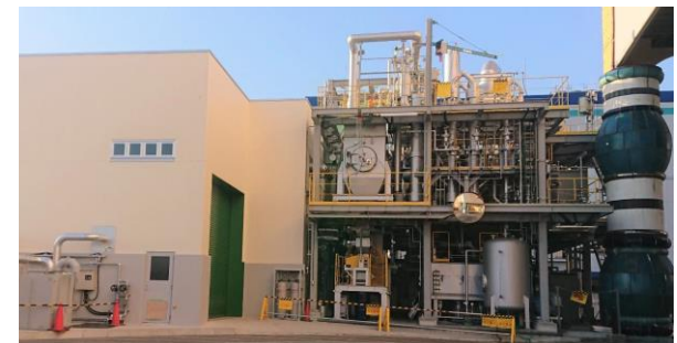
Demonstration plant for Next-Generation Waste Treatment System
