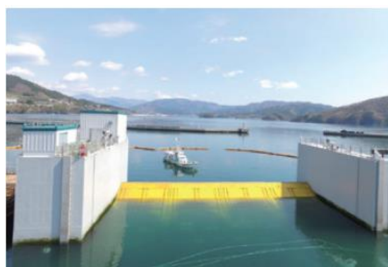
Movable flap-gate type breakwater systems installed on the seabed in Iwate Prefecture (Hosoura Fishing Port)
