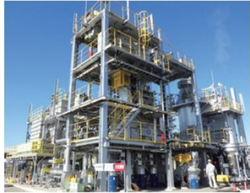
Demonstration test facility (external view)
