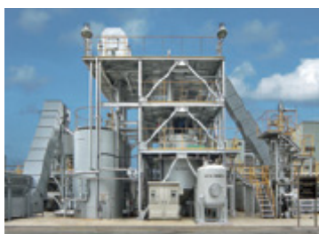
Bioethanol producing plant in “Urban Oil Field” Exploration Project
