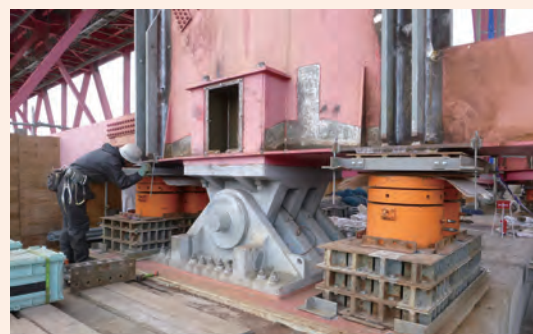
Picture shows reinforcement work being performed on a different bridge in the past.
