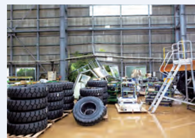
Damaged wall and flooding inside the plant
