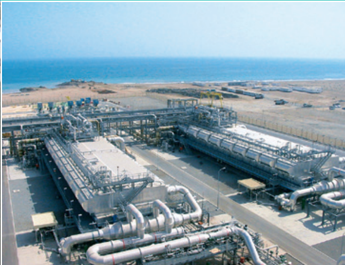
Seawater desalination plant
