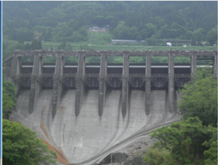
The hydraulic gate Jinzugawa Electric Power Plant
