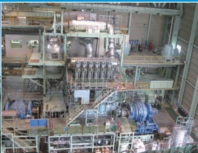
Marine diesel engine fitted with SCR system
