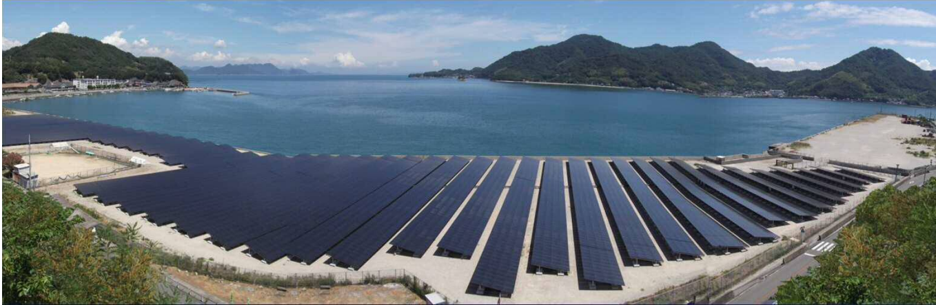
Mega Solar Power Plant 1.5MW, Innoshima works Hiroshima
