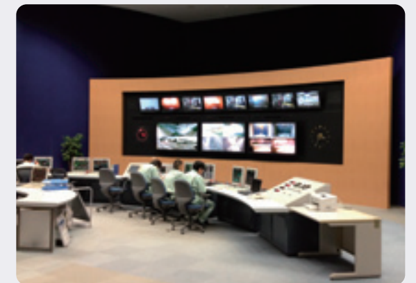
Rinkai Plant Central Control Room
