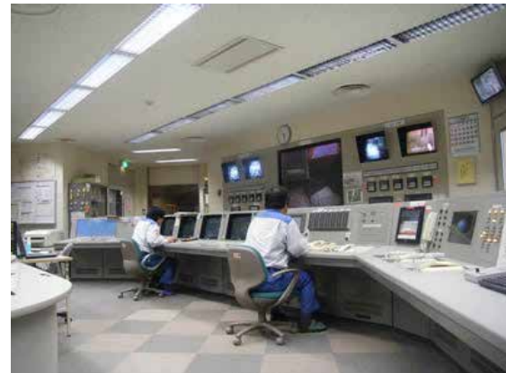
ごみ焼却施設 操作盤 Energy from Waste Plant Operation Panel
