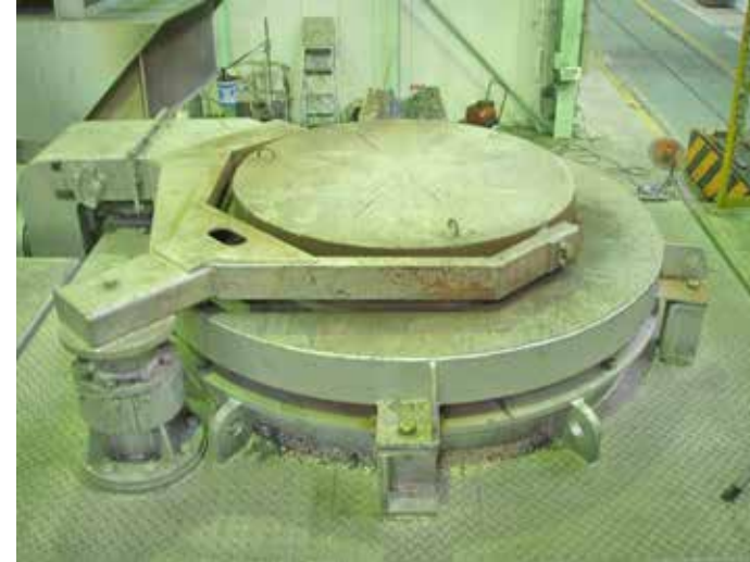
鋳造工場溶解電気炉 Casting Worksite Melting Electric Furnace
