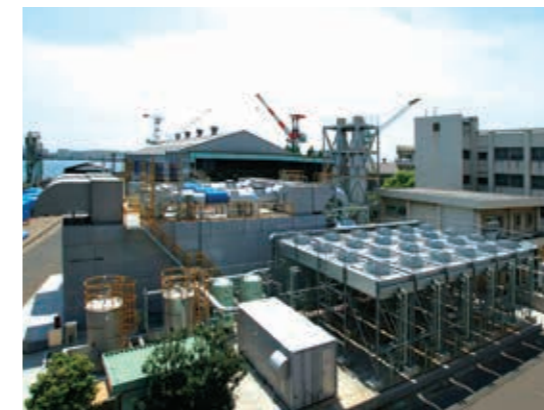
発電所外観 Exterior appearance of power station
