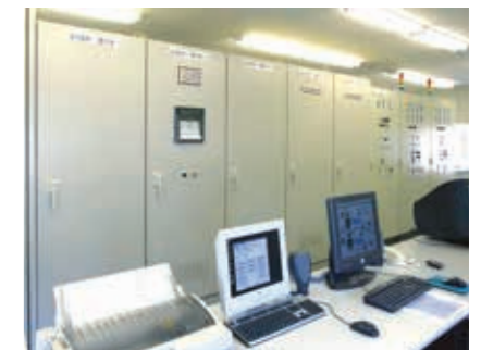
操作室 Control and operation room
