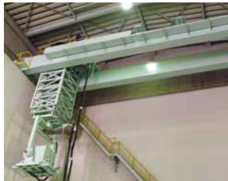
放射線設備 Radiation equipment
