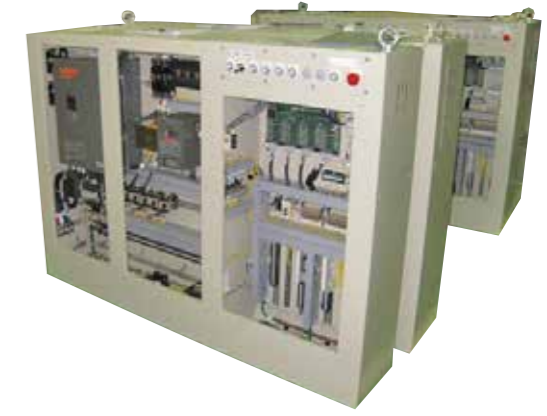
機械式駐車設備 台車動力制御盤 Mechanical Panel Parking Equipment Truck power control board
