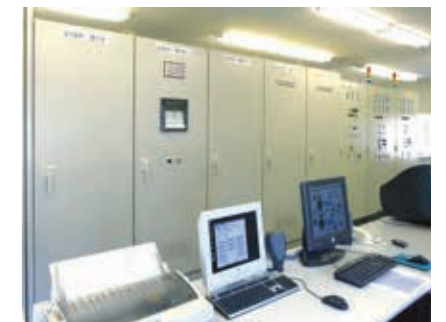
操作室 Control and operation room
