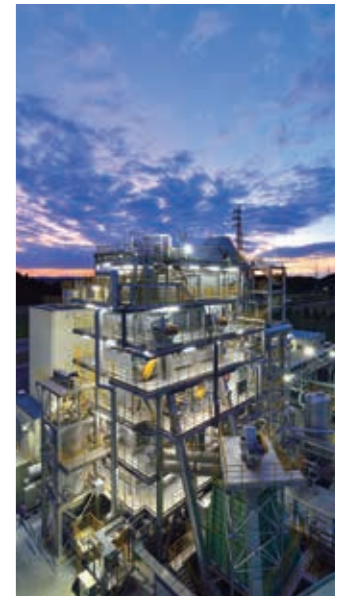
流動床炉ボイラ設備 Fluidized bed furnace boiler
