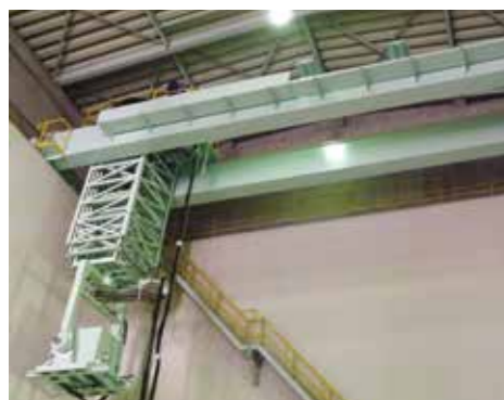
放射線設備 Radiation equipment
