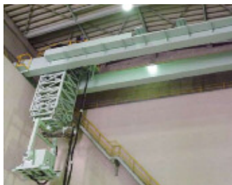
放射線設備 Radiation equipment
